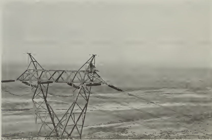
Figure 31. Nesting structure for eagles and other raptors in place on steel transmission tower in Idaho.
